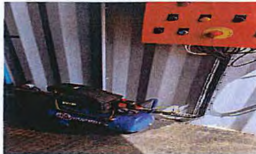
Nkosini Electrical works
