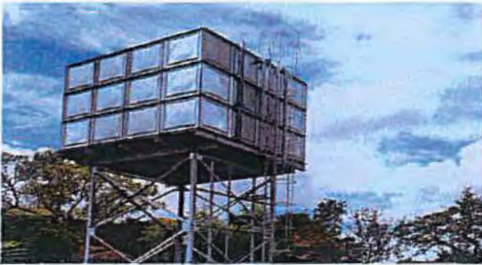
Phokwane / Brooklyn water storage
