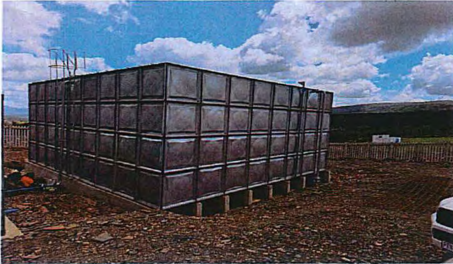
Kgotlopong Steel tank
