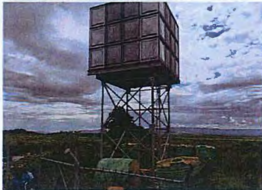
Laersdrift steel tank
